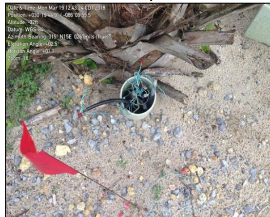
CenturyLink Telephone Pedestal Park Drive; Grayton Beach
