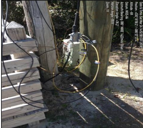
Mediacom Cable TV Aerial Tap Birmingham Street; Seagrove Beach
