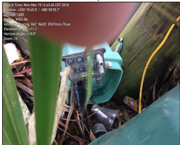
Mediacom Cable TV Pedestal Park Drive; Grayton Beach
