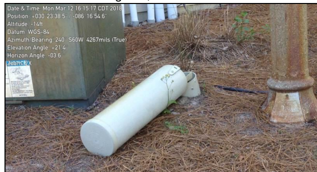
CenturyLink Telephone Pedestal Bald Eagle Ct; Santa Rosa Beach
