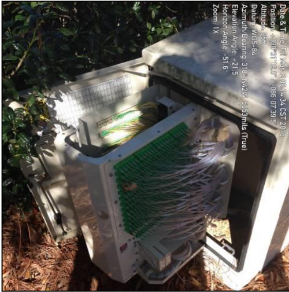
Open CenturyLink Remote Terminal Village Commons Blvd; Freeport
