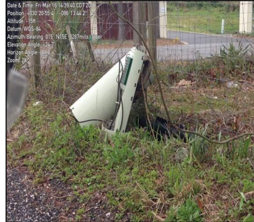
CenturyLink Telephone Pedestal Leisure Lane; Santa Rosa Beach
