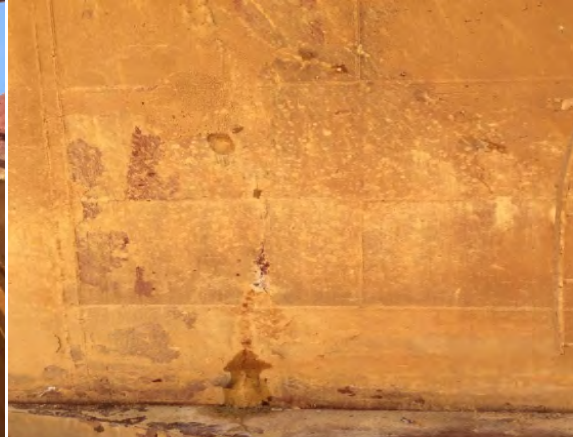
Crack in West Wall of Secondary Settling Basin No. 2.
