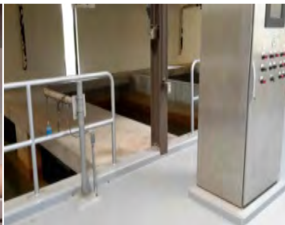
Opening in Guardrail. Recommend this be closed with new safety gate.
