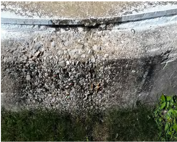
Scaling Due to Erosion of Cement Paste at Base of Wash Water Tower.
