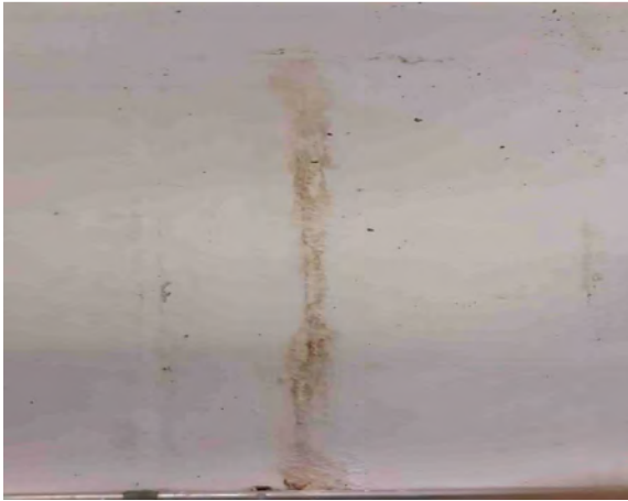
Crack with efflorescence on filter wall. Surface damp to the touch. Typical two locations.
