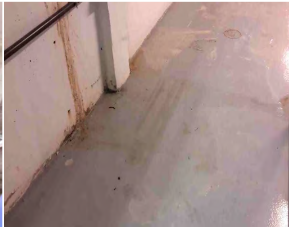
Base of north side expansion joint with water pooling and flowing to floor drain.
