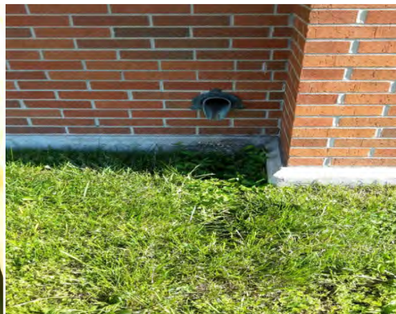
Roof drainage from down spouts drains towards foundation walls.
