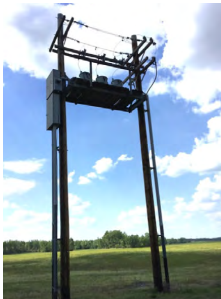
Wells 13, 14 and 15 Service Platform
