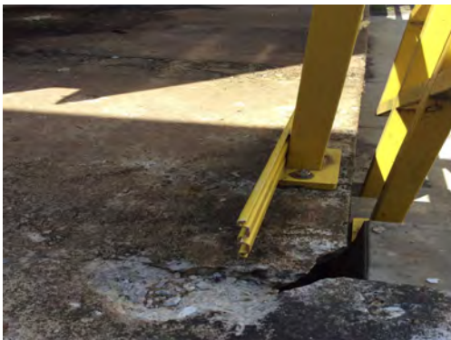
Re-entrant corner with spall and crack.
