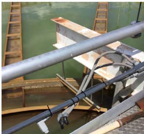
Secondary Basin No. 4 – Abandoned Conduits
