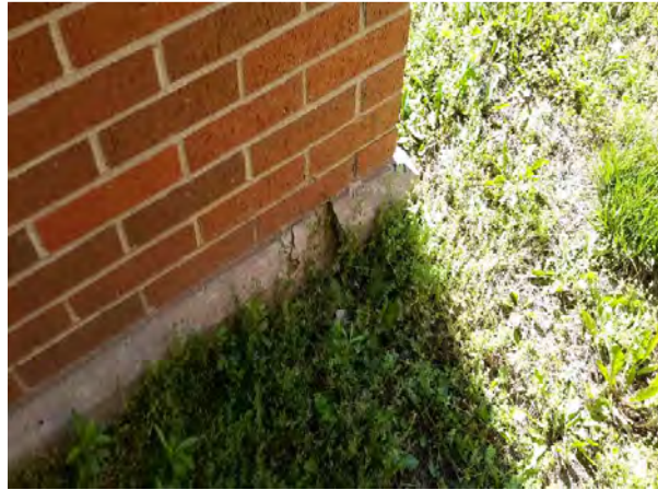
Spall at base of face brick.
