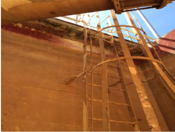
Bent and Damaged Ladder at Secondary Settling Basin No. 2.
