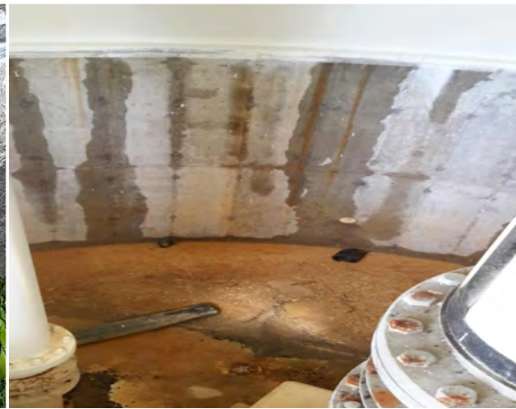
Staining on Interior Surfaces of Tower Foundation Concrete Walls and Base Slab.
