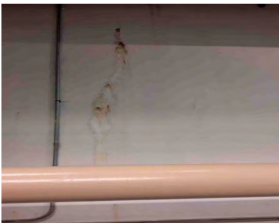
Crack with efflorescence on filter wall. No moisture on surface.
