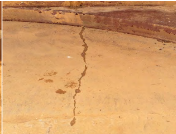
Crack in Base Slab of Secondary Settling Basin No. 2.
