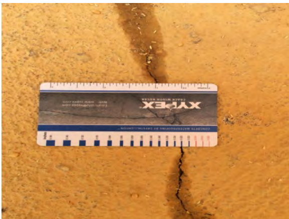
Crack Comparator Measurement of Base slab Crack.
