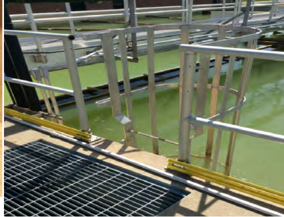
Missing Fall Protection Gate at Ladder (Typical 4 locations) and Conduit Tripping Hazard at Ladder Entry.
