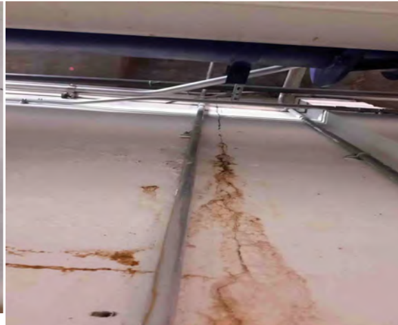
Leaking expansion joint in Filter building Basement.
