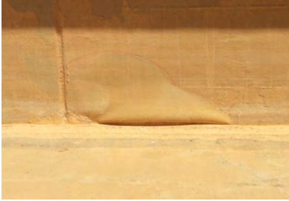
Coating Delamination with Fluid Build Up in Secondary Settling Basin No. 2.
