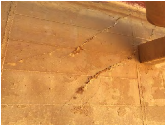
Crack in Southwest corner of West Wall in Secondary Settling Basin No. 2.
