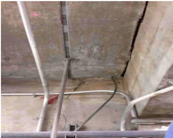
Top of leaking expansion joint. With spalling and cracks.
