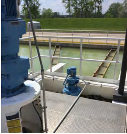
Primary Basin No. 4 - Conduit posing a tripping hazard and subject to damage.
