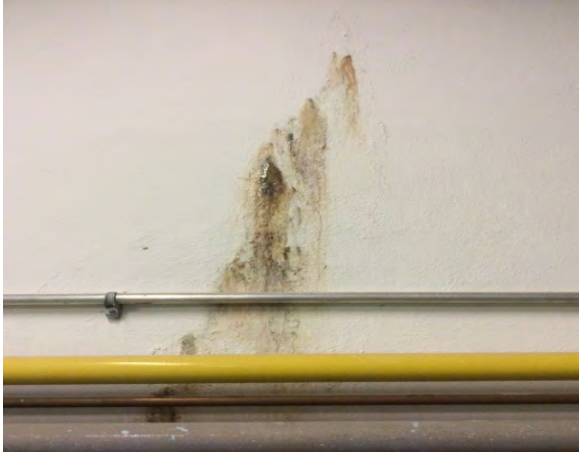
Crack in Tunnel wall.
