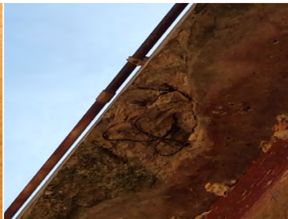
Concrete Spalling at Underside of Walkway on West Side of Secondary Settling Basin No. 2.
