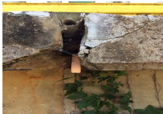
Spalling at construction joint.
