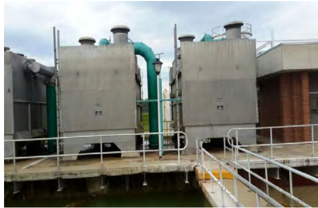
Aerators No. 1 and No. 2
