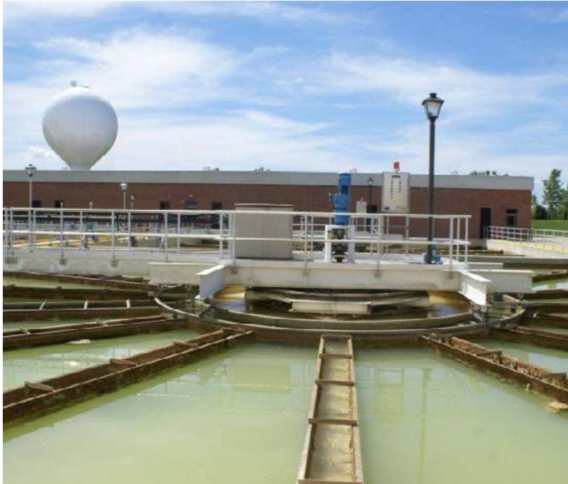
Figure 3-4 McBaine Water Treatment Plant
