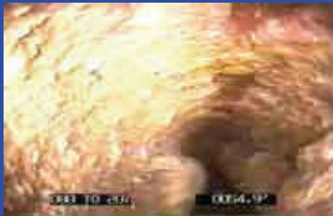
Photo of a Sewer Line clogged with Fats, Oils, and Greases
